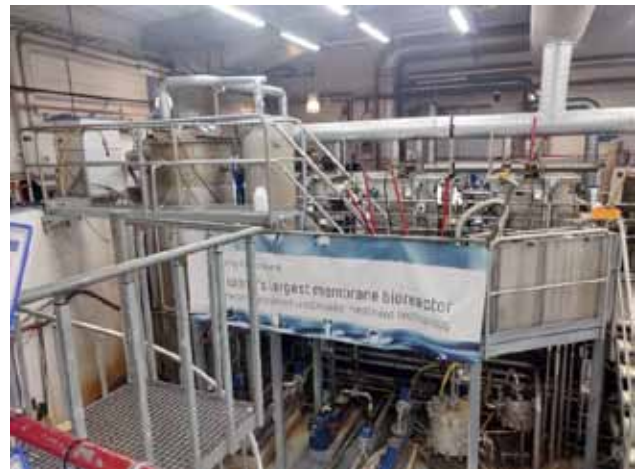
Membrane bioreactor facility of IVL Swedish Environmental Research Institute
